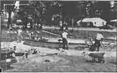
This photo of the current fountain being built appeared in the July 25, 1974 Express. Working on the project were Bader Masonry, Fred Iben, Al Iben, Staner's Plumbing, and REM Electric. (Express photo)
